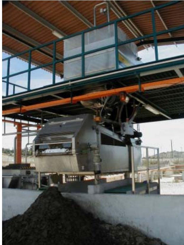
Figure 2: View of Ecopurin separation module installed in at the University of Murcia’s Veterinary School in Spain. Main reactor is in 2 nd floor, filter press is in foreground, and DAF is on the left
