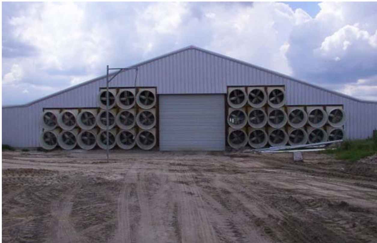
Figure 6. Exhaust fans on tunnel ventilated barn with sprinkler evaporative cooling system.
